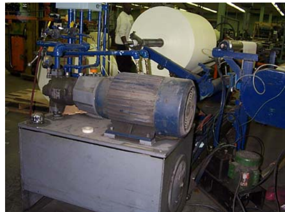
Hydraulic pump, electric motor and reservoir filled with 6110 MONOLEC Hydraulic Oil.
